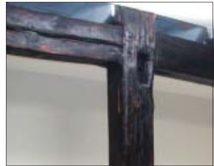
Many beams were charred by the fire. The integrity of the beams was OK, but they had to be cleaned, scraped and sanded, and then varnished to encapsulate the smoke smell.
