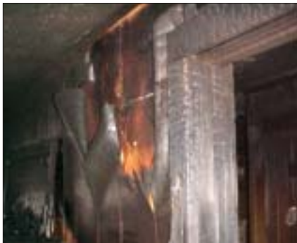
A charred beam after the fire.
