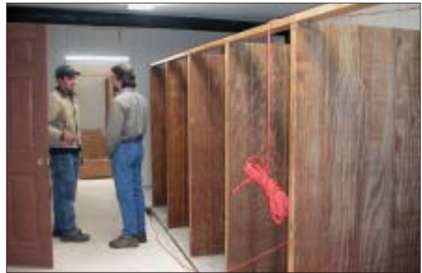
Dr. Nesin talks to J.R. Madden, the lead carpenter for Keith Trembley Builder, in the kennel area.
