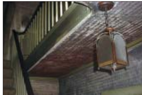
Soot and smoke damage was severe.
