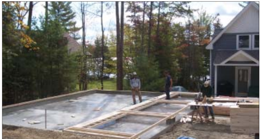
The slab is poured and framing starts to go up on the new oversized garage at the Hews cottage on Sebec Lake. The cottage will be the Hews' retirement home.
