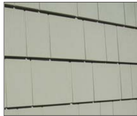
The cedar shake vinyl siding, installed by Ron Michaud, will never have to be painted.
